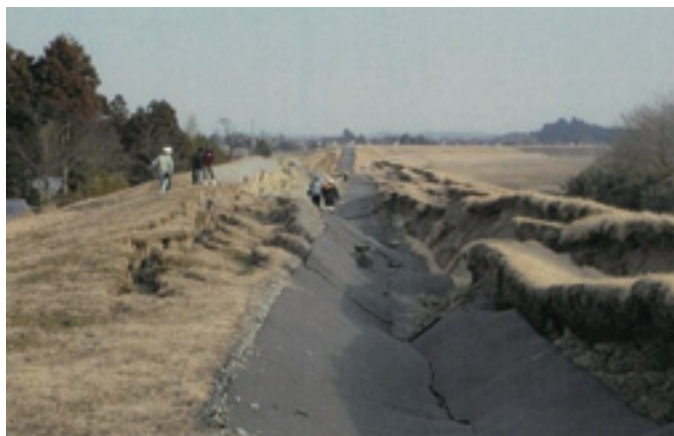
▲鳴瀬川左岸の被災
